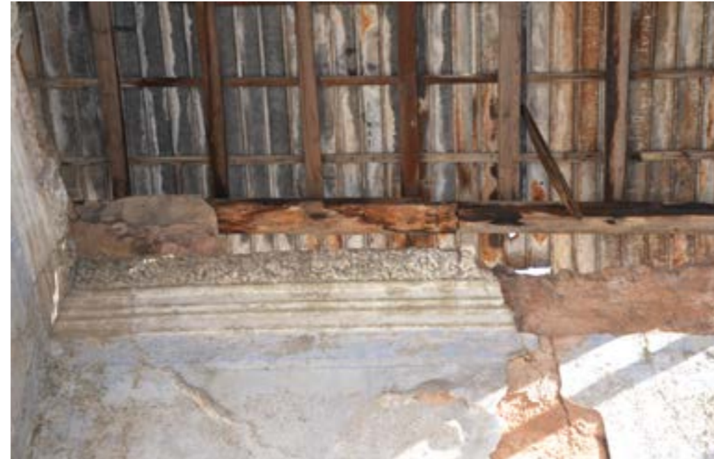
Figure 139 Remnants of hand-carved ceiling finishing were still present in different parts of the mansion.
